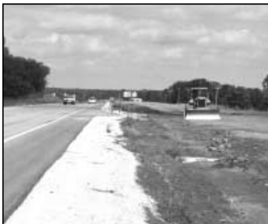
Much of the work this summer on the Quincy to Macomb leg was from north of Mendon to Loraine.
